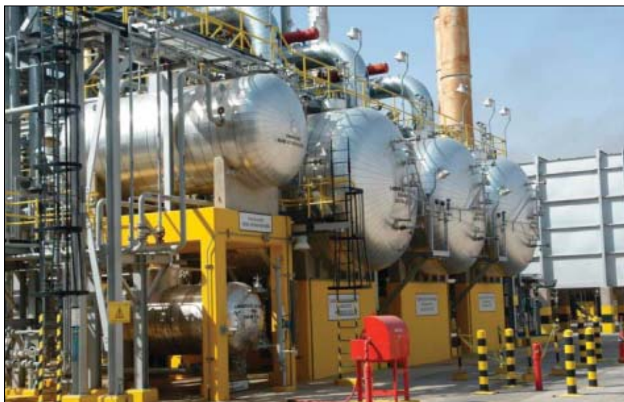
In the left foreground of this view of one of the carbon units, the regeneration condensate three-phase separator sits above the condensate-collection drum. To the right of these are the three carbon-adsorption-bed vessels (Fig. 3).
